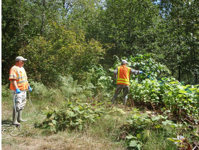
Grandy Creek roadside before treatment.
