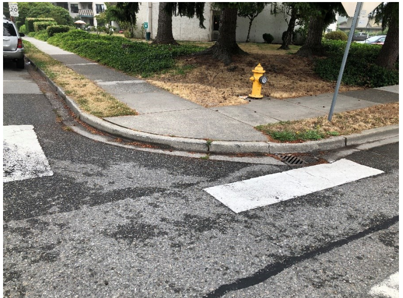
ADA Barriers include missing curb ramps at crosswalks such as these at the intersection of State Street and Township Street.
